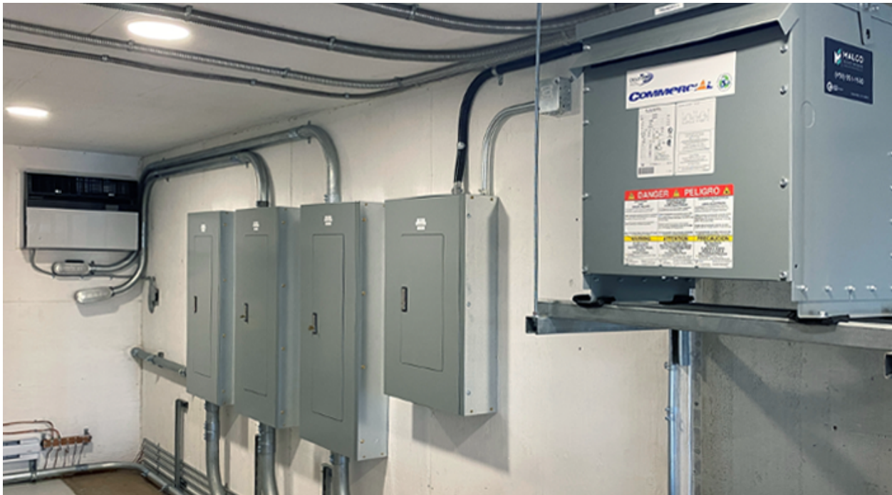
FIGURE 11 • Autobus Maheux’s updated building electrical room to power the charging infrastructure
