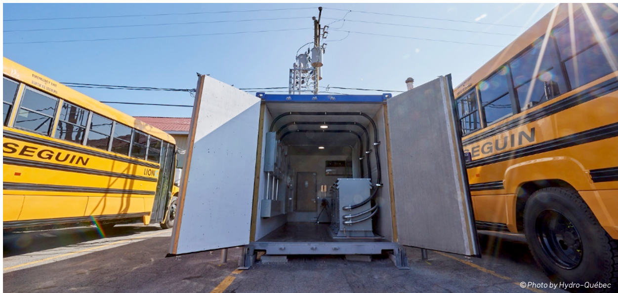
FIGURE 5 • Installation by Cléo of a container for Autobus Séguin bus capable of supplying up to twelve 260 kW charging stations
